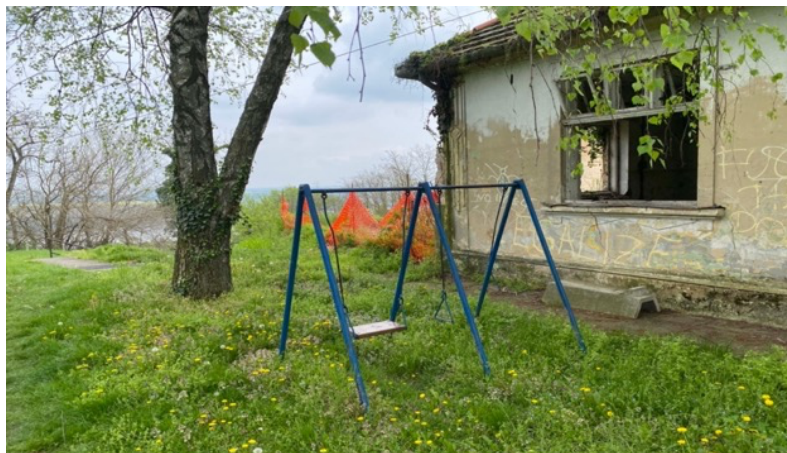
Swing set beside an abandoned and damaged house in Erdut, Baranja county.
